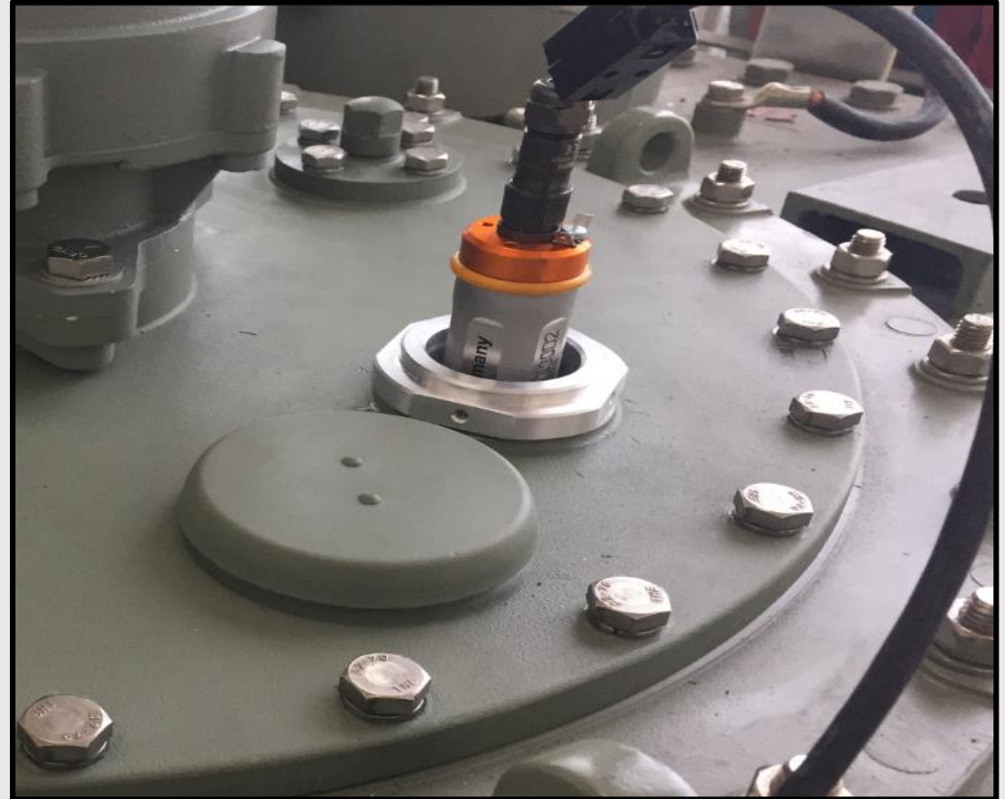
Mounting on top of Tapchanger
