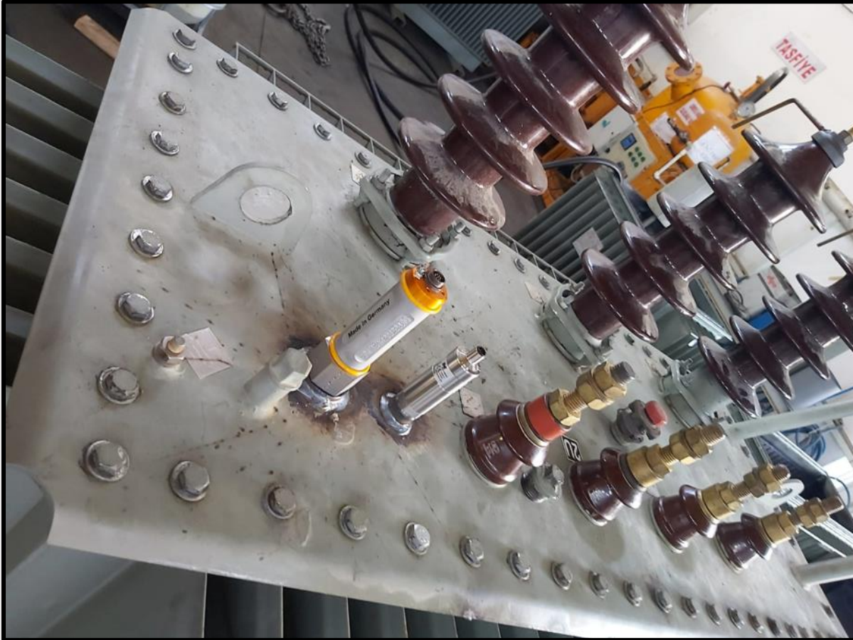
Mounting on top of transformer tank
