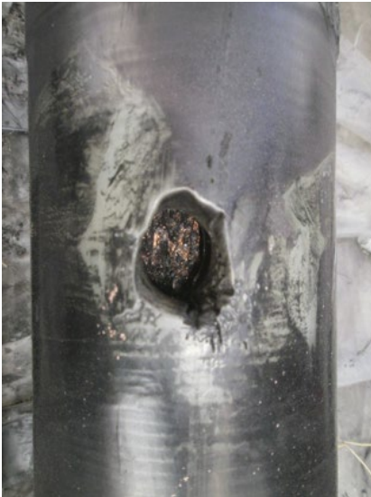
Insulation breakdown at a cable termination
